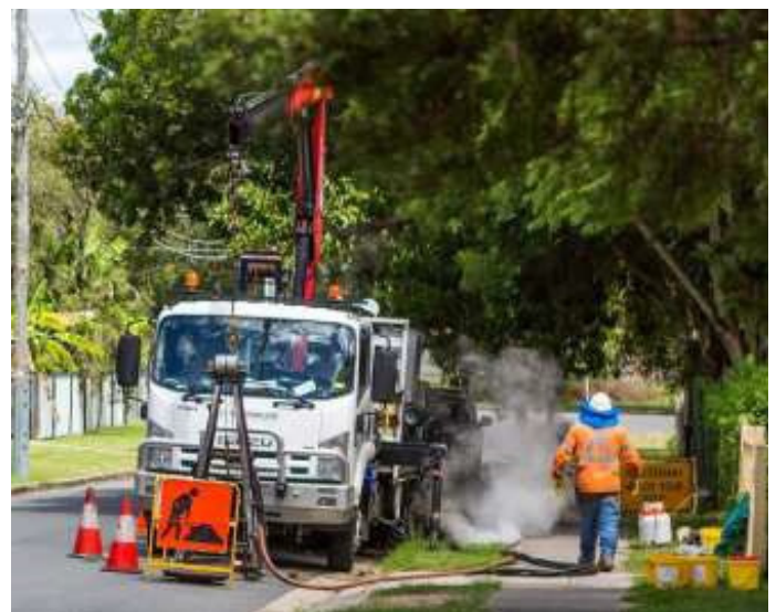
Abergeldie uses steam to cure a new liner in a section of pipeline.
